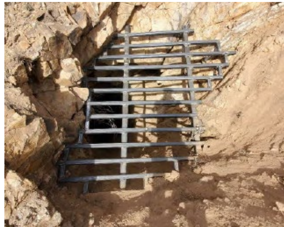
Bat friendly grate installed at Golden Idol
